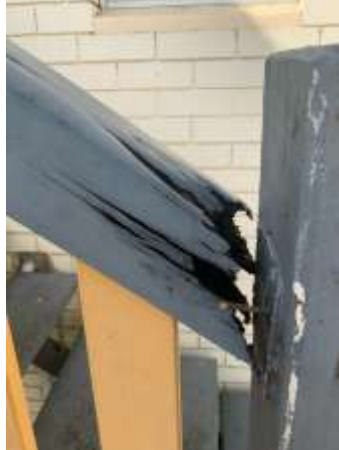
Showing evidence of Fungal Decay
