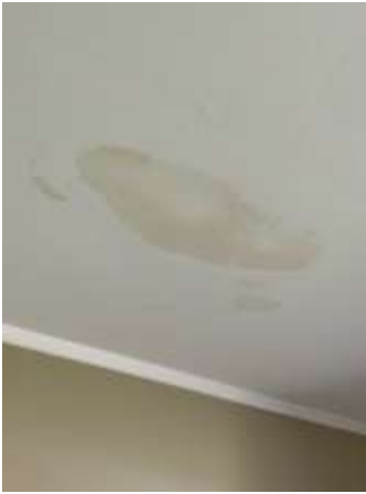
Moisture/mould staining to ceiling, recommend engaging a Roofer to fix the upper roof to reduce the risk of water leaks from roof coverings, penetration & flashings
