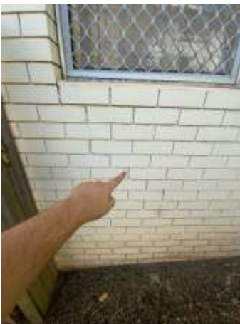
Movement cracking with Diagonal, Vertical, Horizontal pattern noted on the external wall, specifically around openings. A Structural Engineer should be consulted for further evaluation and advice prior to your purchase of the property.
