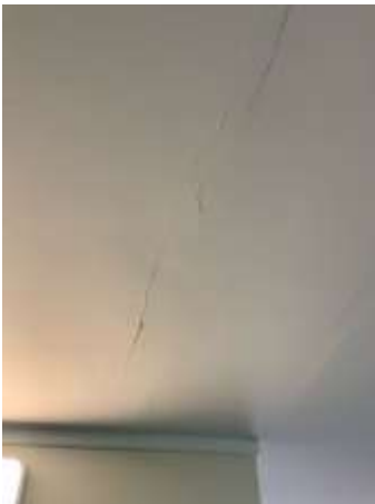
Sagging and Creasing visible on ceiling plasterboards, Recommend repair by engaging a licensed Plasterer.
