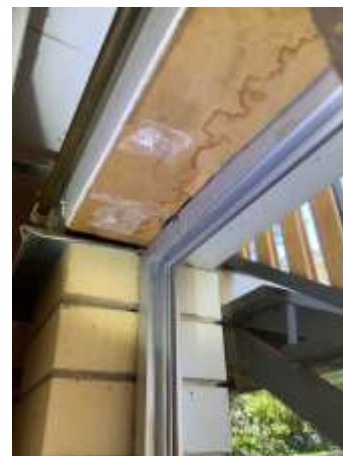
Water damage noted to window reveal, recommend proper sealing around window and replacing affected Timbers.
