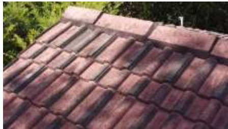
Few chipped and dislocated tiles noted to roof exterior coverings, recommend engage a roofer to rectify.
