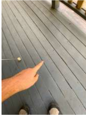
Ageing and weathering to the Timber decking including handrails/balustrades and floorboards, recommend repair/replacing damaged Timbers ASAP.
