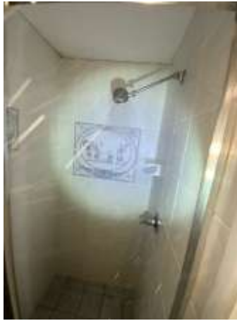
High moisture reading to walls adjacent to the Bathroom / Shower recess-Recommend engaging a Builder for further invasive investigation to ascertain cause and to determine if there is any concealed damage to the timber framing., Downstairs Bathroom
