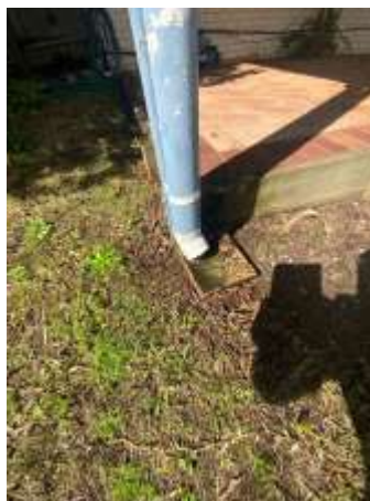
Few Downpipes damaged/cracked/dismounted or not properly connected to stormwater system- Recommend engaging a Plumber to repair & avoid the risk of foundation movement & other moisture related issues.
