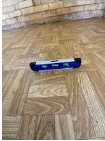
Undulating/uneven floors - recommend engaging a Builder to assess appropriate method of rectification to prevent further deterioration.
