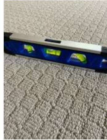
Undulating/uneven floors - recommend engaging a Builder to assess appropriate method of rectification to prevent further deterioration.
