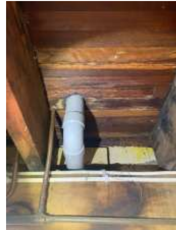
Signs of water damage to Timber flooring, especially around pipe penetration. Engage a Builder for further assessment and repair proposals.
