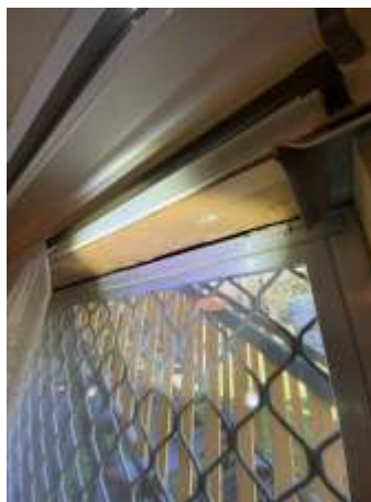
Water damage noted to window reveal, recommend proper sealing around window and replacing affected Timbers.
