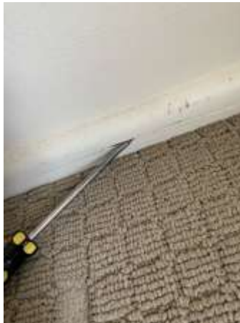
Termite damage noted to the Wall Skirting in Bedroom 2, Highly recommend engage a Builder for further investigation to determine the extent of damage and repair proposals.
