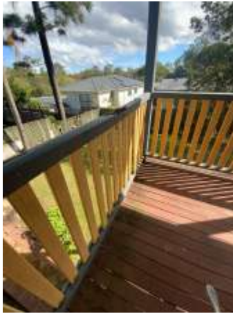
Showing evidence of Timber Safety Hazard
