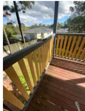
Showing evidence of Fungal Decay
