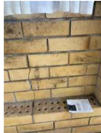
Diagonal crack patterns around openings, Due to the extent, pattern & width of cracks, highly advise to consult with a Licensed Structural Engineer.
