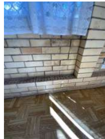
Diagonal crack patterns around openings, Due to the extent, pattern & width of cracks, highly advise to consult with a Licensed Structural Engineer.
