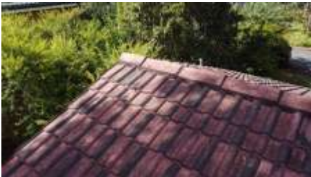
Few chipped and dislocated tiles noted to roof exterior coverings, recommend engage a roofer to rectify.
