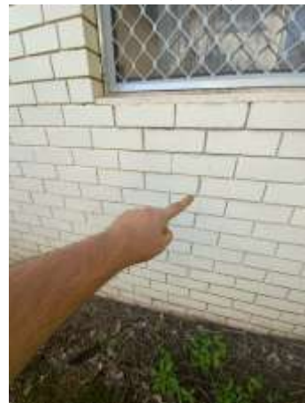
Movement cracking with Diagonal, Vertical, Horizontal pattern noted on the external wall, specifically around openings. A Structural Engineer should be consulted for further evaluation and advice prior to your purchase of the property.
