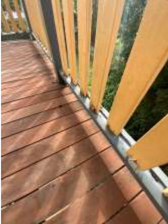
Showing evidence of Timber Safety Hazard
