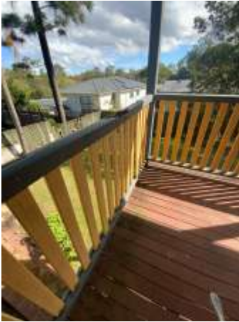
Ageing and weathering to the Timber decking including handrails/balustrades and floorboards, recommend repair/replacing damaged Timbers ASAP.
