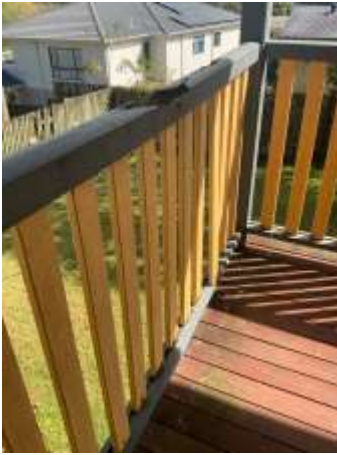
Showing evidence of Fungal Decay
