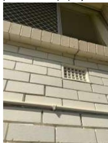
Movement cracking with Diagonal, Vertical, Horizontal pattern noted on the external wall, specifically around openings. A Structural Engineer should be consulted for further evaluation and advice prior to your purchase of the property.
