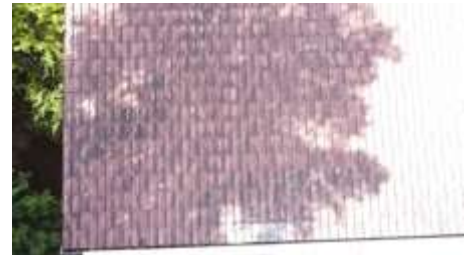
Few chipped and dislocated tiles noted to roof exterior coverings, recommend engage a roofer to rectify.
