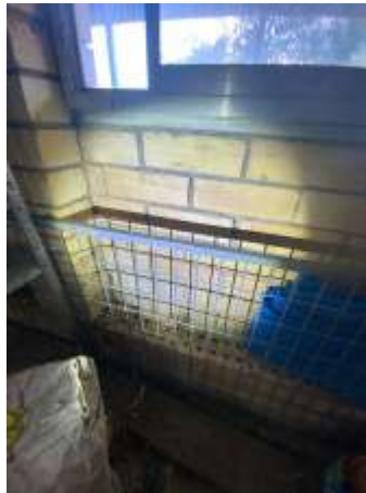
Diagonal crack patterns around openings, Due to the extent, pattern & width of cracks, highly advise to consult with a Licensed Structural Engineer.
