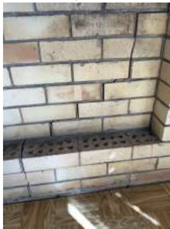
Diagonal crack patterns around openings, Due to the extent, pattern & width of cracks, highly advise to consult with a Licensed Structural Engineer.
