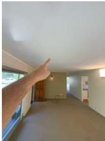
Sagging and Creasing visible on ceiling plasterboards, Recommend repair by engaging a licensed Plasterer.
