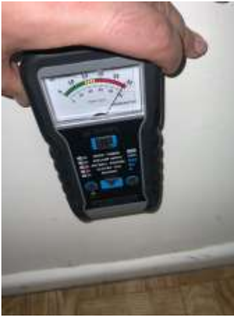
High moisture reading to walls adjacent to the Bathroom / Shower recess-Recommend engaging a Builder for further invasive investigation to ascertain cause and to determine if there is any concealed damage to the timber framing., Downstairs Bathroom
