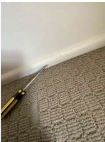
Termite damage noted to the Wall Skirting in Bedroom 2, Highly recommend engage a Builder for further investigation to determine the extent of damage and repair proposals.
