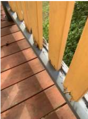
Showing evidence of Fungal Decay
