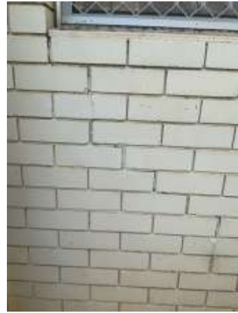
Movement cracking with Diagonal, Vertical, Horizontal pattern noted on the external wall, specifically around openings. A Structural Engineer should be consulted for further evaluation and advice prior to your purchase of the property.
