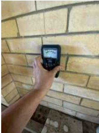
Signs of rising damp to the Brick walls to the Garage, recommend improving the surface drainage behind the wall.
