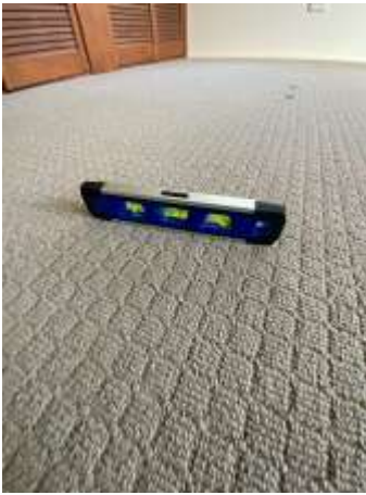
Undulating/uneven floors - recommend engaging a Builder to assess appropriate method of rectification to prevent further deterioration.
