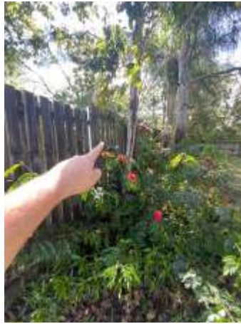
Leaning fences to parts - recommend engaging a Builder or Fencer to rectify to prevent further deterioration.
