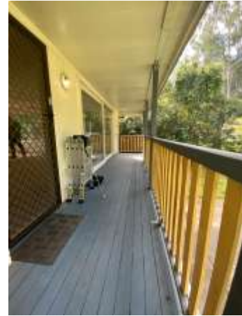
Ageing and weathering to the Timber decking including handrails/balustrades and floorboards, recommend repair/replacing damaged Timbers ASAP.
