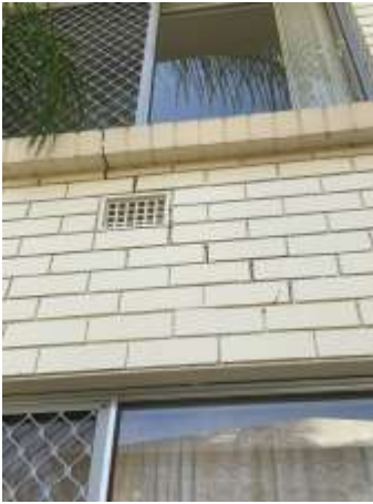
Movement cracking with Diagonal, Vertical, Horizontal pattern noted on the external wall, specifically around openings. A Structural Engineer should be consulted for further evaluation and advice prior to your purchase of the property.
