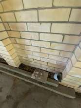
Signs of rising damp to the Brick walls to the Garage, recommend improving the surface drainage behind the wall.
