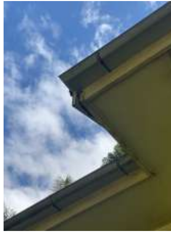
Aged, weathered and deteriorated fascia/ridge - needs repair/replacing.
