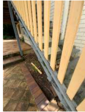
Showing evidence of Fungal Decay
