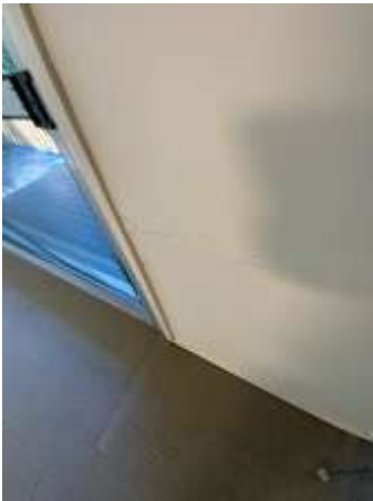
Common crack to parts of Internal walls (Fluctuations in temperature and humidity levels can cause framing members and drywall to expand and contract, resulting in cracking). Repair by engaging a licensed Plasterer / Painter.
