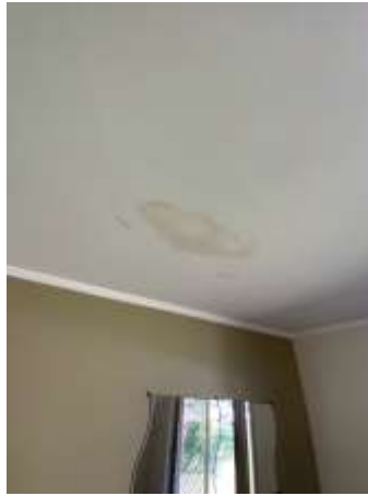
Moisture/mould staining to ceiling, recommend engaging a Roofer to fix the upper roof to reduce the risk of water leaks from roof coverings, penetration & flashings
