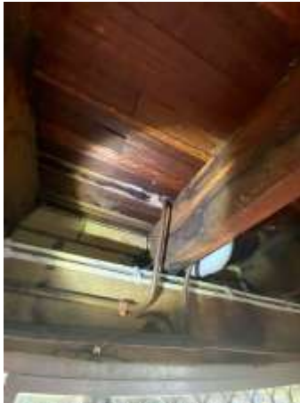
Signs of water damage to Timber flooring, especially around pipe penetration. Engage a Builder for further assessment and repair proposals.
