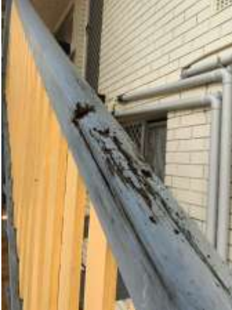
Showing evidence of Fungal Decay
