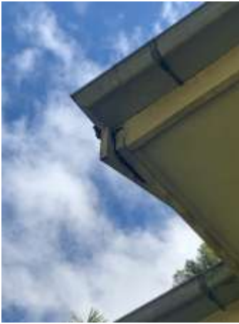
Aged, weathered and deteriorated fascia/ridge - needs repair/replacing.
