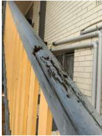
Ageing and weathering to the Timber decking including handrails/balustrades and floorboards, recommend repair/replacing damaged Timbers ASAP.
