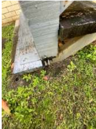
Ageing and weathering to the Timber decking including handrails/balustrades and floorboards, recommend repair/replacing damaged Timbers ASAP.
