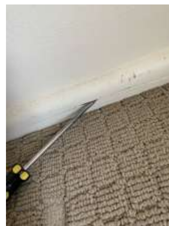
Showing evidence of Termite Workings
