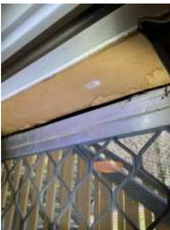
Water damage noted to window reveal, recommend proper sealing around window and replacing affected Timbers.
