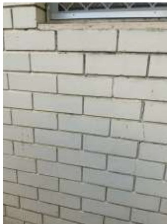
Movement cracking with Diagonal, Vertical, Horizontal pattern noted on the external wall, specifically around openings. A Structural Engineer should be consulted for further evaluation and advice prior to your purchase of the property.
