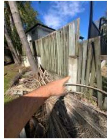
Concrete block boundary walls leaning to parts, recommend engage a Builder to rectify.
