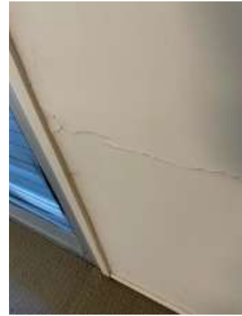
Common crack to parts of Internal walls (Fluctuations in temperature and humidity levels can cause framing members and drywall to expand and contract, resulting in cracking). Repair by engaging a licensed Plasterer / Painter.
