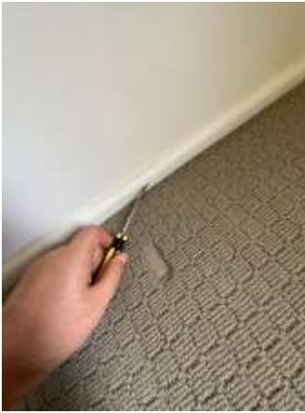
Showing evidence of Termite Workings
