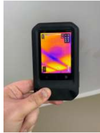
Moisture/mould staining to ceiling, recommend engaging a Roofer to fix the upper roof to reduce the risk of water leaks from roof coverings, penetration & flashings
