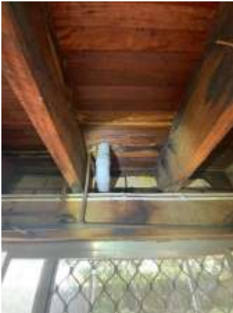
Signs of water damage to Timber flooring, especially around pipe penetration. Engage a Builder for further assessment and repair proposals.
