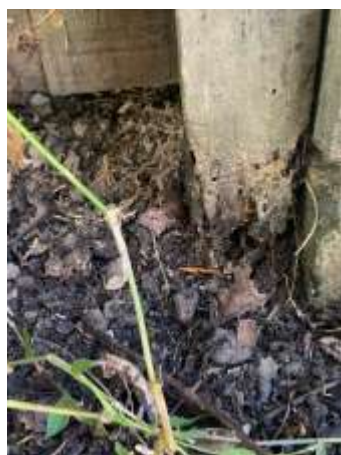
Showing evidence of Termite Workings
