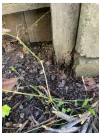
Showing evidence of Termite Workings
