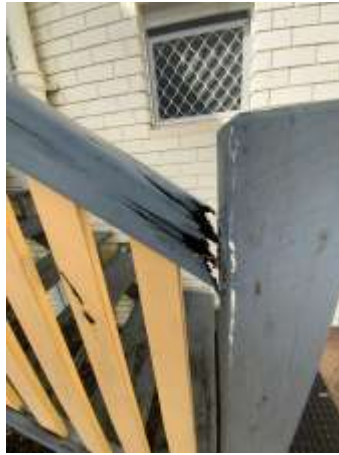
Showing evidence of Fungal Decay
