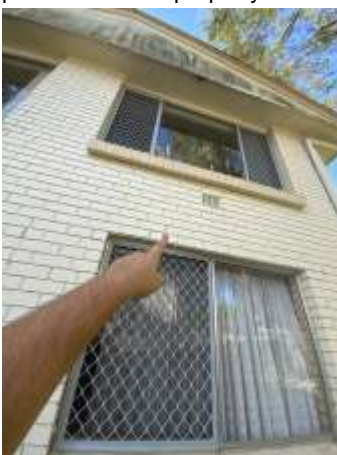
Movement cracking with Diagonal, Vertical, Horizontal pattern noted on the external wall, specifically around openings. A Structural Engineer should be consulted for further evaluation and advice prior to your purchase of the property.
