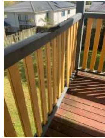
Ageing and weathering to the Timber decking including handrails/balustrades and floorboards, recommend repair/replacing damaged Timbers ASAP.
