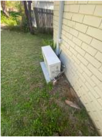
Showing samples of Excessive Moisture
