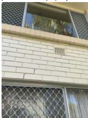
Movement cracking with Diagonal, Vertical, Horizontal pattern noted on the external wall, specifically around openings. A Structural Engineer should be consulted for further evaluation and advice prior to your purchase of the property.
