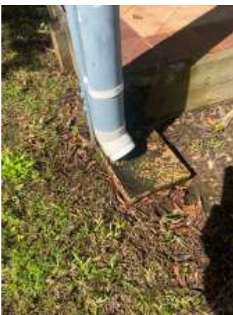
Few Downpipes damaged/cracked/dismounted or not properly connected to stormwater system- Recommend engaging a Plumber to repair & avoid the risk of foundation movement & other moisture related issues.
