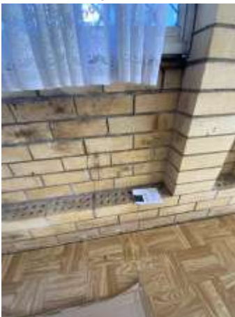
Diagonal crack patterns around openings, Due to the extent, pattern & width of cracks, highly advise to consult with a Licensed Structural Engineer.
