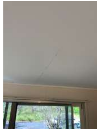
Sagging and Creasing visible on ceiling plasterboards, Recommend repair by engaging a licensed Plasterer.
