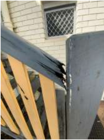
Ageing and weathering to the Timber decking including handrails/balustrades and floorboards, recommend repair/replacing damaged Timbers ASAP.
