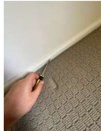
Termite damage noted to the Wall Skirting in Bedroom 2, Highly recommend engage a Builder for further investigation to determine the extent of damage and repair proposals.
