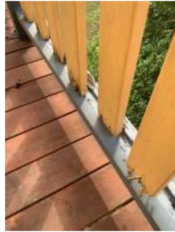
Showing evidence of Timber Safety Hazard
