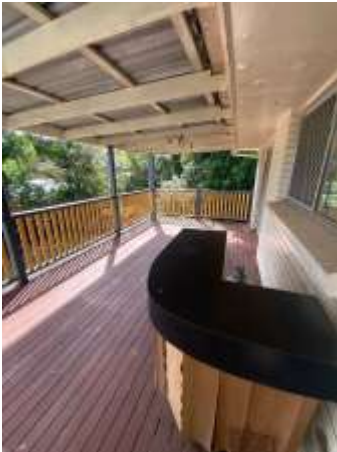
Ageing and weathering to the Timber decking including handrails/balustrades and floorboards, recommend repair/replacing damaged Timbers ASAP.
