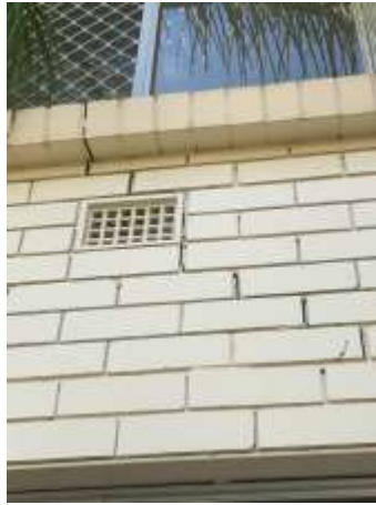
Movement cracking with Diagonal, Vertical, Horizontal pattern noted on the external wall, specifically around openings. A Structural Engineer should be consulted for further evaluation and advice prior to your purchase of the property.
