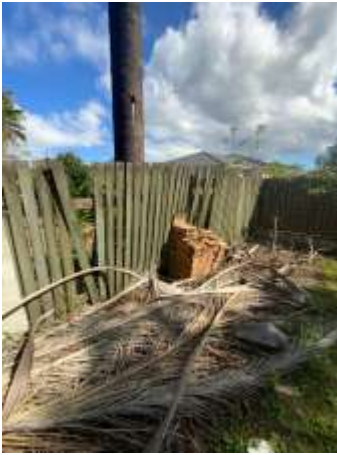
Leaning fences to parts - recommend engaging a Builder or Fencer to rectify to prevent further deterioration.
