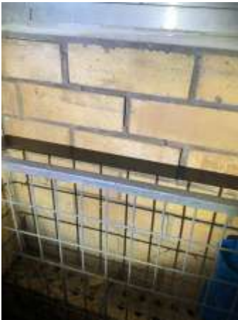
Diagonal crack patterns around openings, Due to the extent, pattern & width of cracks, highly advise to consult with a Licensed Structural Engineer.
