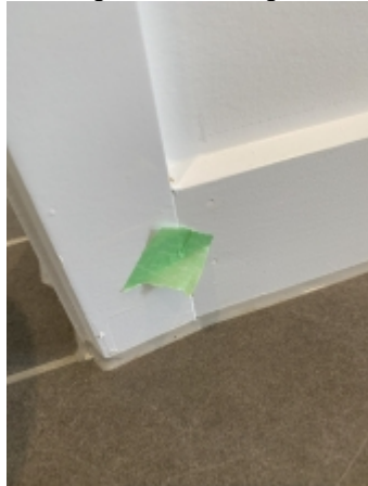
Showing defects throughout the property
