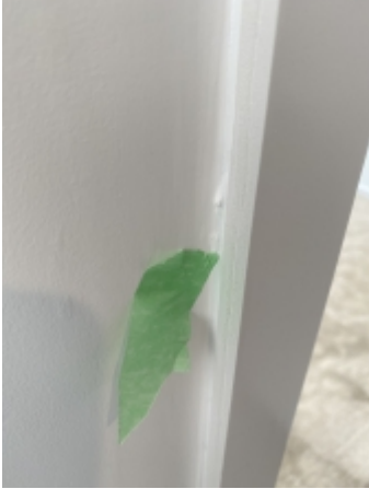
Showing defects throughout the property
