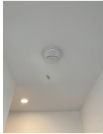
Showing defects throughout the property
