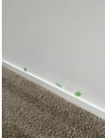
Showing defects throughout the property
