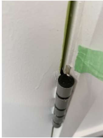
Showing defects throughout the property
