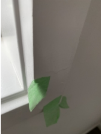
Showing defects throughout the property
