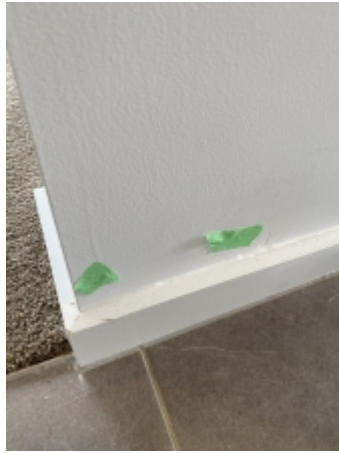
Showing defects throughout the property
