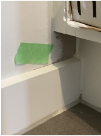
Showing defects throughout the property
