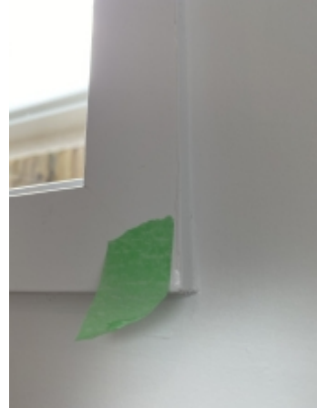
Showing defects throughout the property
