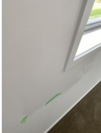
Showing defects throughout the property
