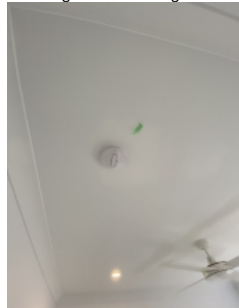
Showing defects throughout the property
