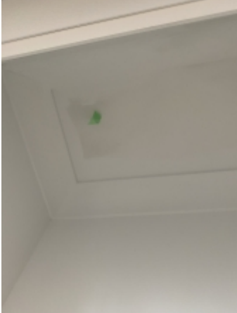
Showing defects throughout the property
