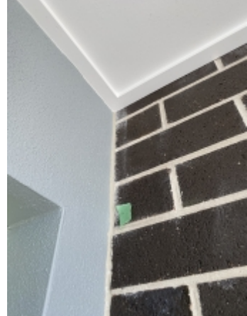
Showing defects throughout the property
