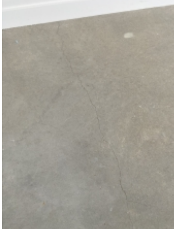
Showing defects throughout the property
