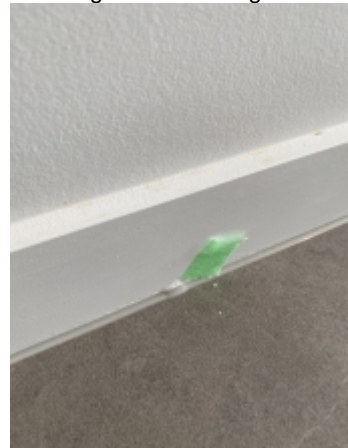
Showing defects throughout the property
