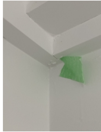
Showing defects throughout the property
