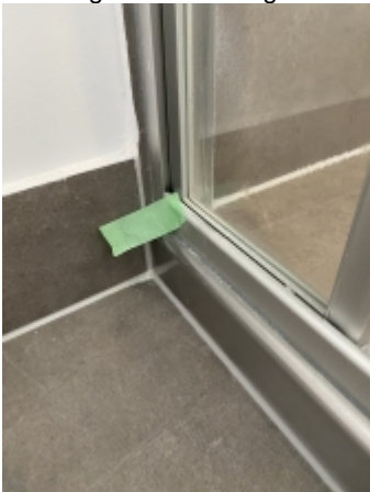
Showing defects throughout the property
