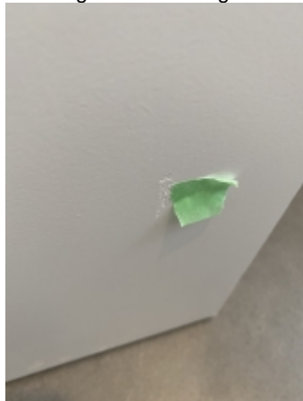
Showing defects throughout the property
