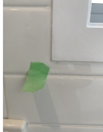
Showing defects throughout the property
