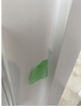
Showing defects throughout the property
