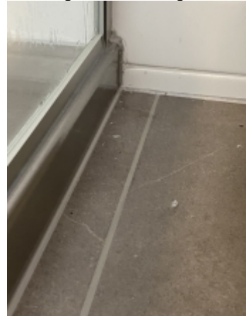
Showing defects throughout the property
