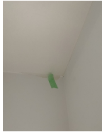
Showing defects throughout the property
