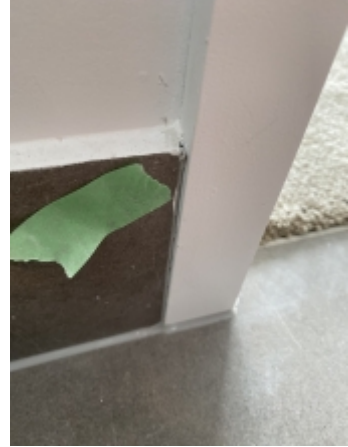
Showing defects throughout the property
