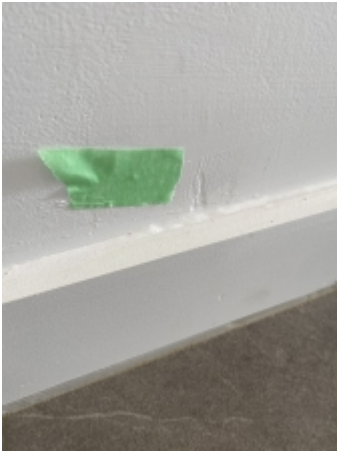
Showing defects throughout the property
