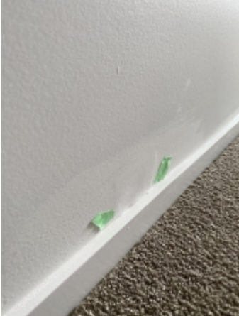
Showing defects throughout the property
