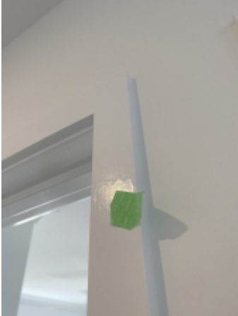
Showing defects throughout the property
