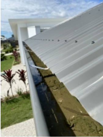
Showing defects throughout the property
