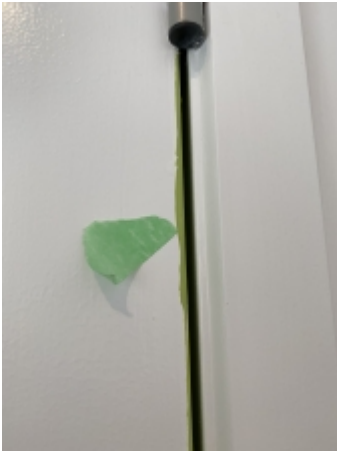
Showing defects throughout the property
