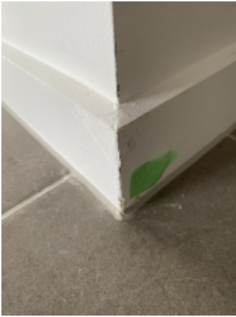
Showing defects throughout the property
